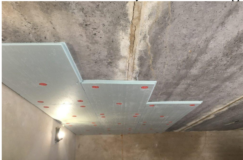
Fig. 3. Thermal insulation of the basement and first floor ceilings before thermal modernization
