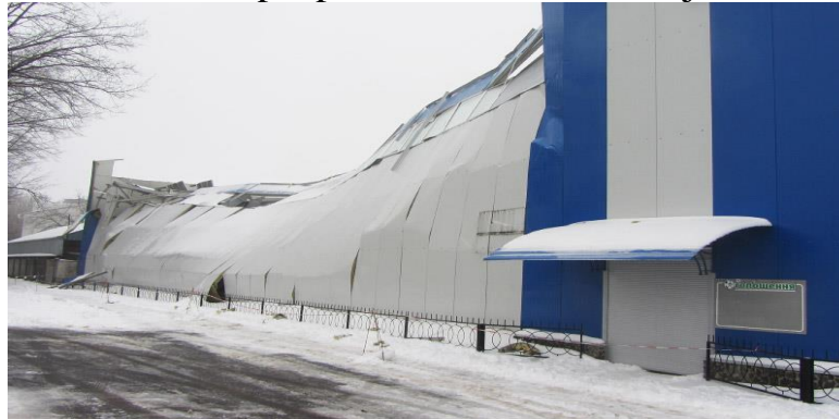
Fig.1. A sports complex collapsed on Komarova St. in Poltava, Ukraine
